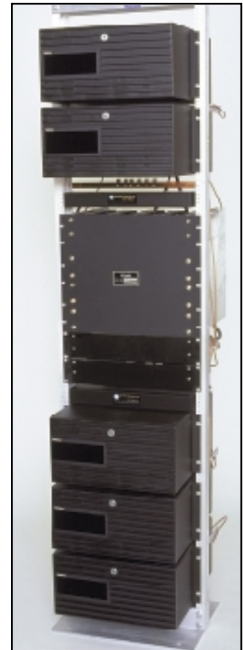
Five Channels and 7-Foot Rack
