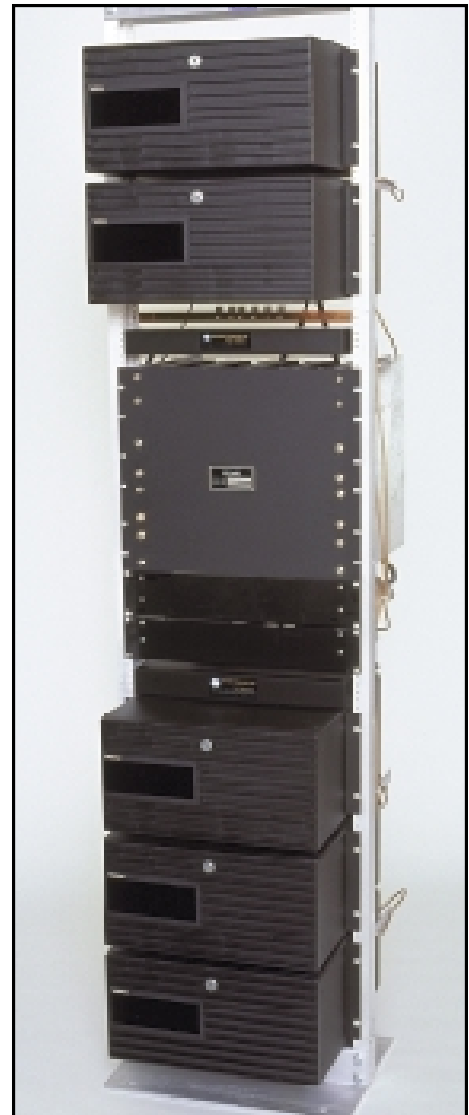
Five Channels and 7-Foot Rack
