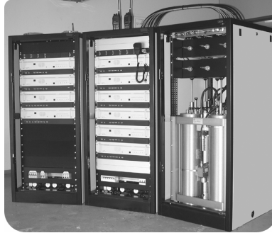
Figure 7-2 MX800 Setup in system rack
